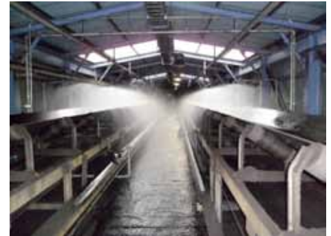
The PLC immediately stops the conveyor belt and activates the sprinkler system when the temperature alarm is triggered.
