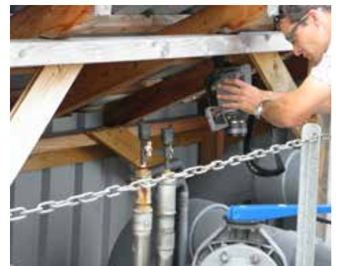
Engineer Ibeling van Lessen looking for gas leaks, which is possible from a safe distance and unusual angles using the FLIR GF320.
