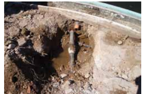
The repair workers were directed to open up the pavement where leaks were inspected, to find broken or cracked pipework, validating the results from the thermographic survey.
